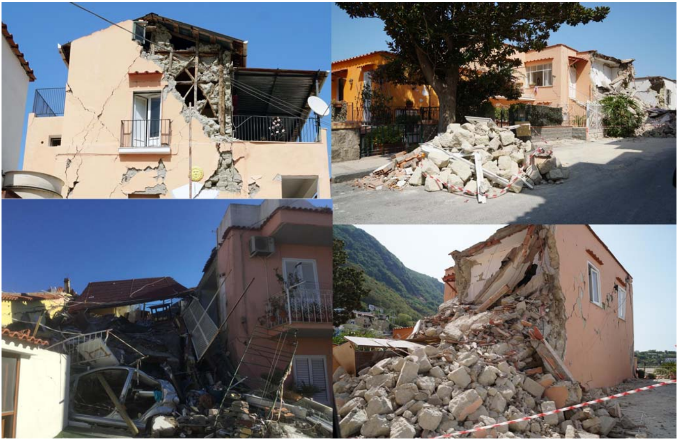
▲ Figure 2. Houses collapsed and heavily damaged by the 21 August 2017 earthquake in the hilly historical center of Casamicciola Terme (Ischia island). Photos by S. Porfido. The color version of this figure is available only in the electronic edition.
