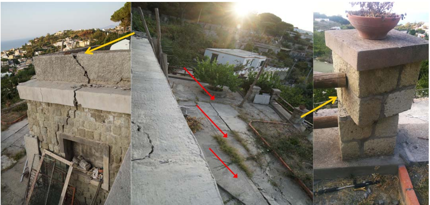
▲ Figure 5. Coseismic ruptures (the arrows in the middle picture) cutting ground, road pavement and man-made structures along Montecito road (middle picture from stop 60 to 70 in Table S1); the arrows pointing toward right and left indicate two details of the middle picture: on the right rotated pillar is shown, on the left the man-made structures fractured (Fig. 3 for location). The color version of this figure is available only in the electronic edition.
