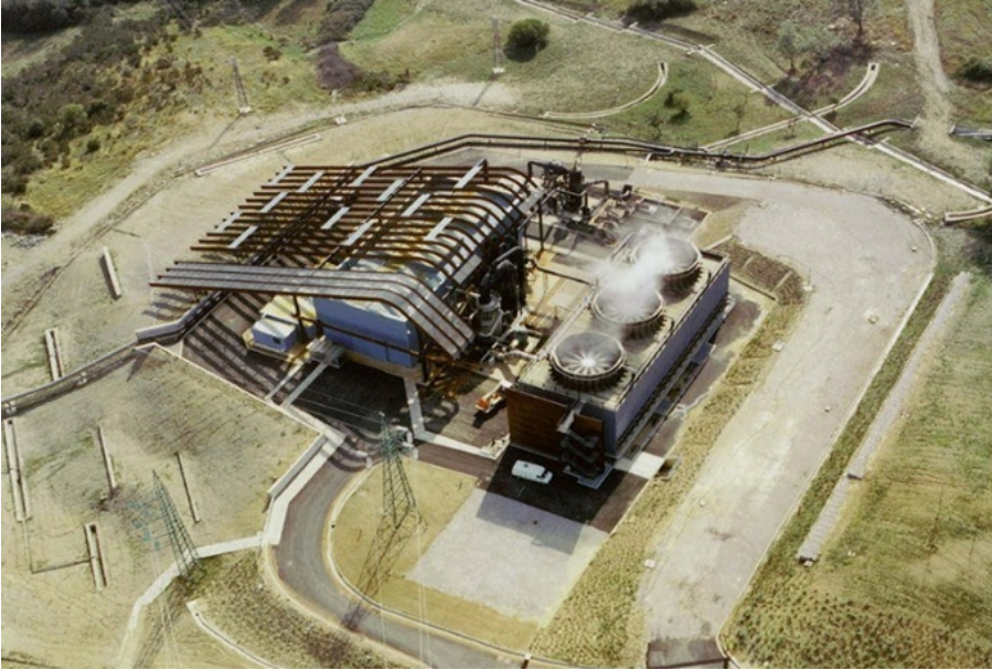
Figure 6. Bagnore 3 power plant, top view (photo by Fabio Sartori)
